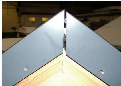
Figure 10 – The second section is lowered to meet the first section at the apex
