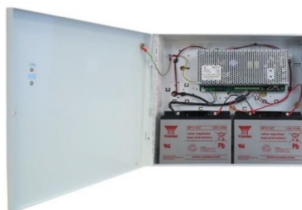
Figure 7 – Battery backup supply
